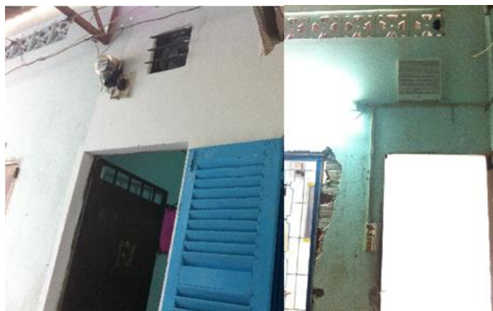
(c) The sample house underwent renovation with the installation of a new window and an exhaust fan
