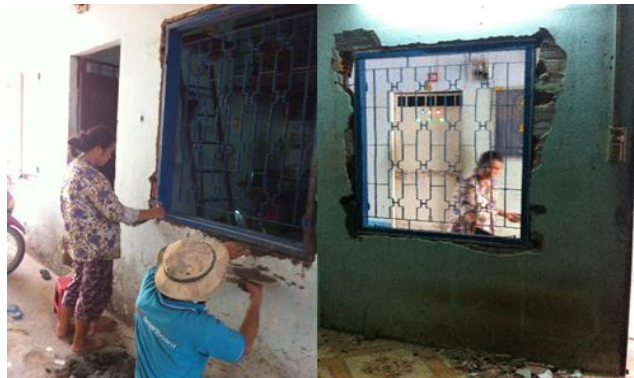
(b) Upgrade and Replace the Previous Window. The new window was a type of louvered window that has fixed horizontal slats to allow for air to flow through
