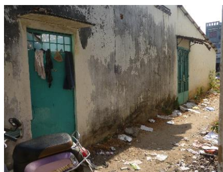
(f) The soil surrounding the house was not paved with concrete.
