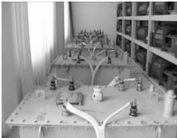
Figure 7 The single-phase three-winding transformers
